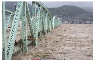
Flood water surging over Kumano-ohashi Bridge
