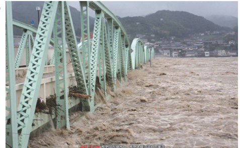
Flood water surging over Kumano-ohashi Bridge
