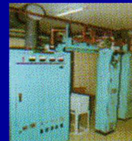
Water Level supervisory equipment
