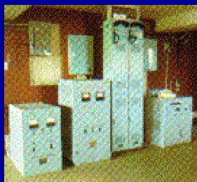
Rainfall Supervisory equipment
