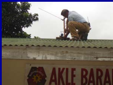
Installation of Rain gauge Gauge
